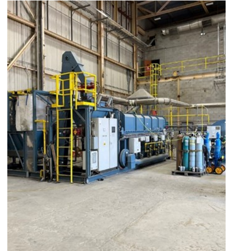
Photo of Pyrolysis Kiln at CHAR facility
